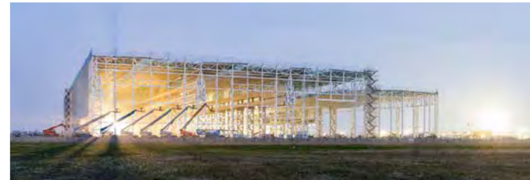
The production hall and all the auxiliary buildings had to be ready for production in only 10 months
